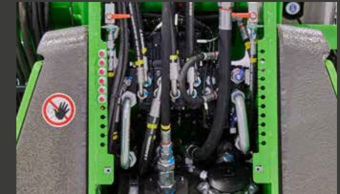
6 Best possible access to the main manifold, hydraulic oil tank and return filter.
